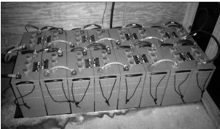
Sixteen deep-cycle batteries for storage of energy generated by solar panels.
